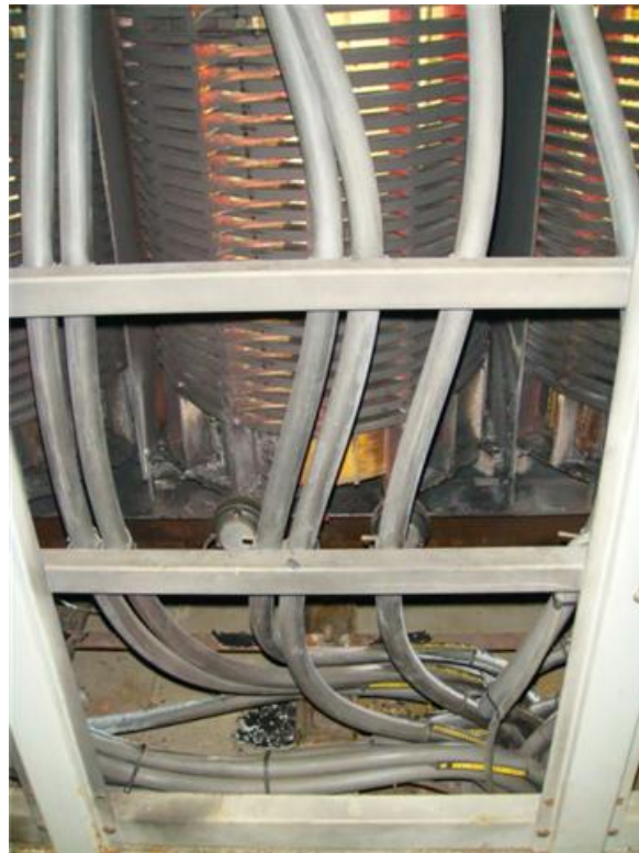
Insulation system failure
